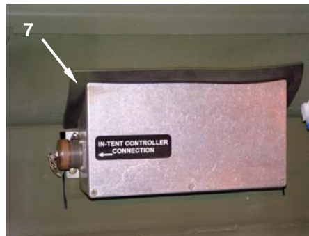
Figure 1. SHC-60K Installed Outside of Tent.
